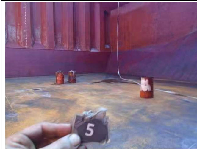
View of condition in Hold No.5
