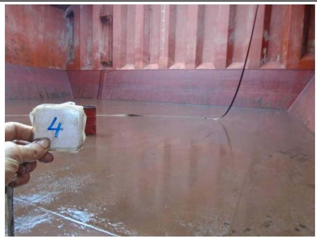
View of condition in Hold No.4
