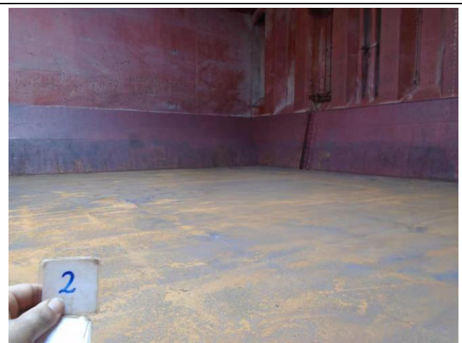
View of condition in Hold No.2
