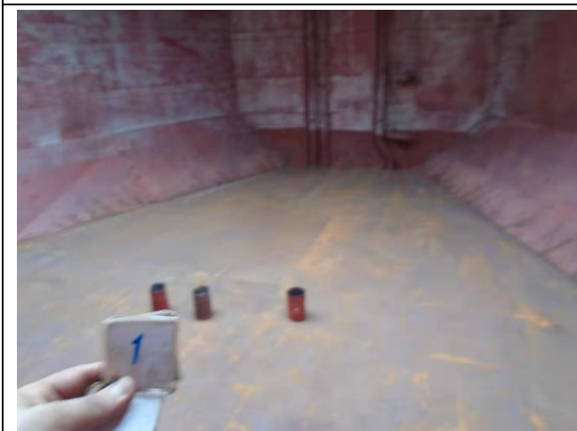
View of condition in Hold No.1
